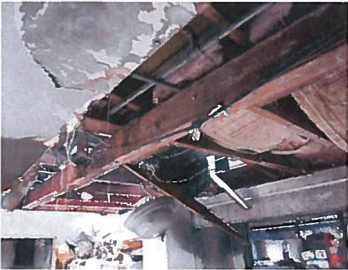
Area of non-permitted addition
