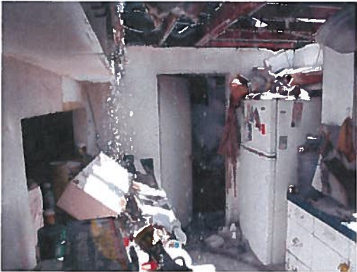
Area of non-permitted addition
