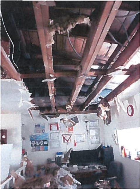
Area of non-permitted addition
